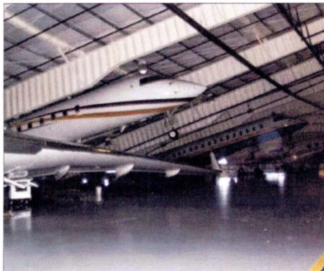
The collapsed roof at Dulles Jet Center in Washington, D.C. Insurance companies faced a bill for millions of dollars in damages after a massive snowstorm hit the U.S. East Coast in February 2010.
